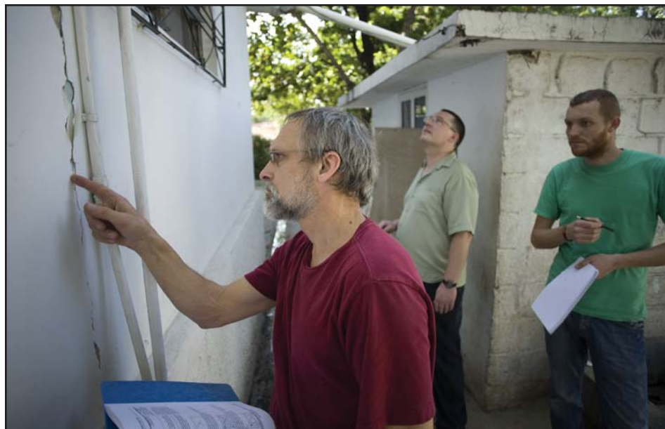
Johann Zimmermann (left) inspects a crack in a building wall with other engineers .
