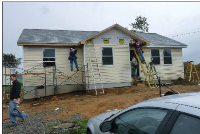
Volunteers putting up siding at a storm-damaged home. Photo courtesy of Richard Rhodes.
