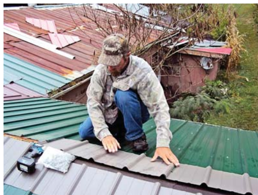
A member of the Grace Mennonite team works on a new metal roof. Photos courtesy of Karin King
