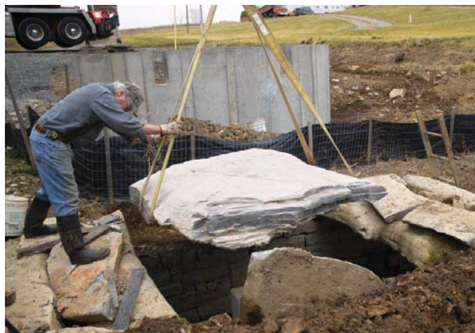
A worker guides the lifting of a stone slab weighing over three tons to allow for more excavation. Photos courtesy of author
