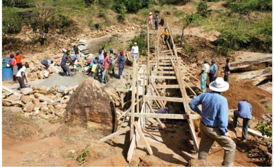
Team members Deryl Kennel (with back to the camera), Ralph Swartzentruber (white t-shirt and hat), and Joan Chamberlain (pink shirt and hat) with a view of the forms in an early phase of dam construction. Photos courtesy of author
