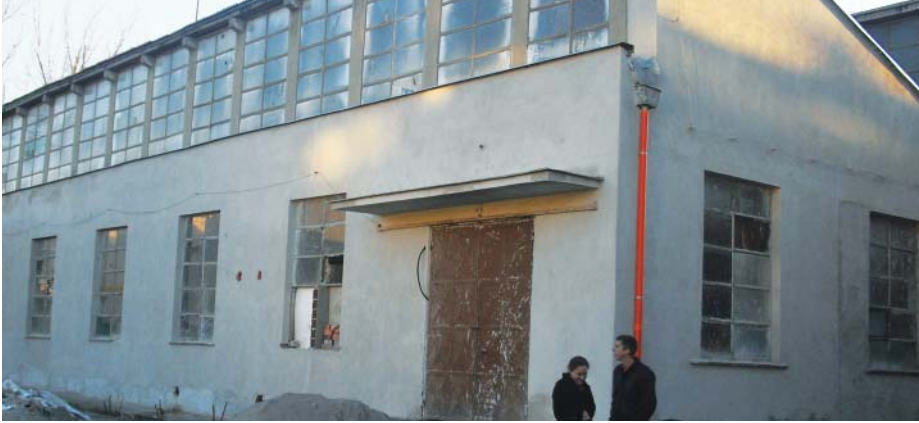
Rachel and Kris Bucher stand outside the warehouse being renovated for the milk plant. Courtesy of author
