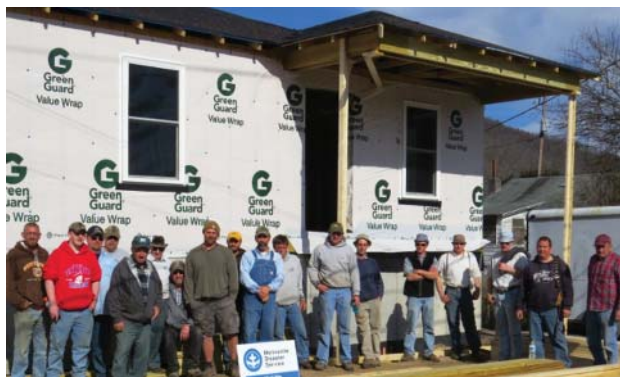
The new home build, along with a large volunteer framing group, for the Rex family in Rainelle, West Virginia. The home owner is on the left hand side. Photo by Rod Burkholder
